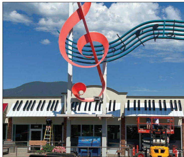
Salmon Arm's Spectrum Signworks began installing a new metal awning at Shuswap Park Mall on Lakeshore Drive last Friday, July 22. A portion of the awning behind the giant treble clef sculpture was designed to look like a piano keyboard. (Spectrum Signworks photo)
